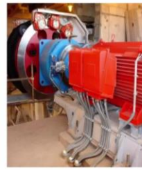
Driving station of RopeCon
